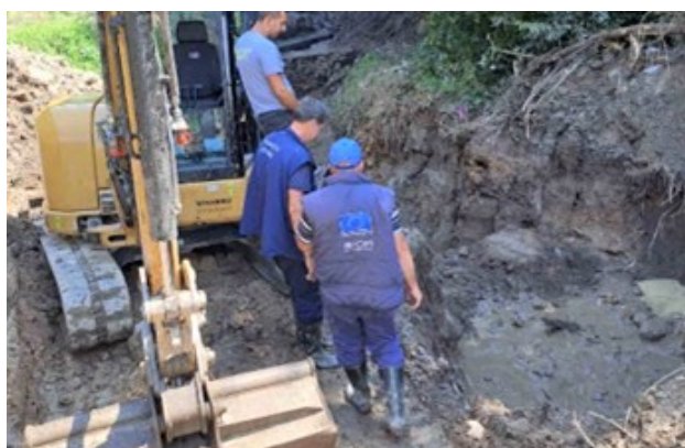
INSTALLATION OF WATER PIPES IN TRC UŠIVAK TO ENSURE AN ADEQUATE DRAINAGE SYSTEM. ©IOM 2023
